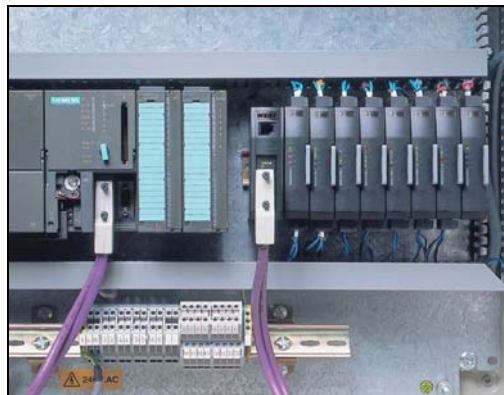
MLC 9000+ Installed System
